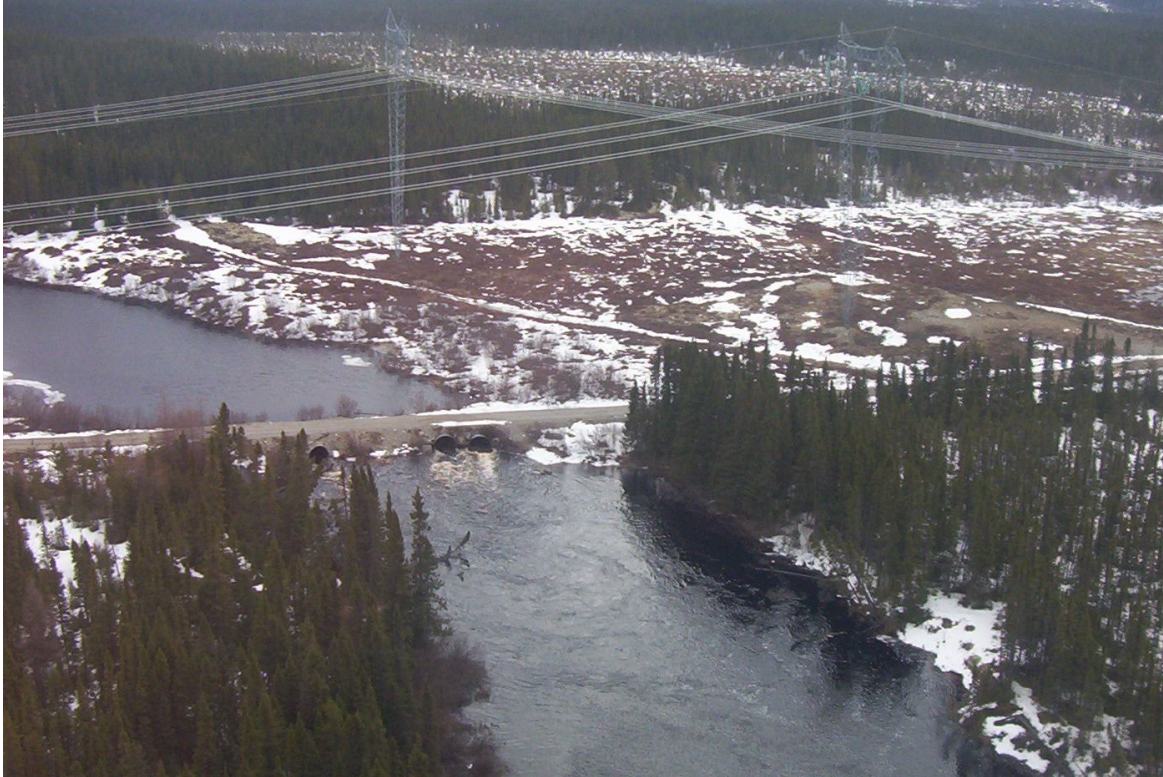
Photo 8.1: Water crossing dating back to the construction of Hydro-Québec's power transmission line. This crossing will need to be completely replaced by a bridge built according to current standards.
